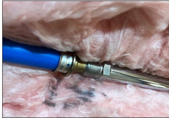
Figure 9.47 Insulated Hydrant to Prevent Freezing
