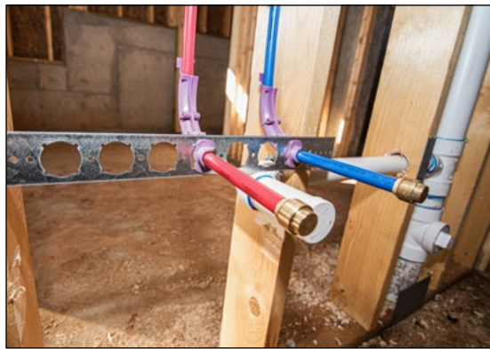
Figure 9.43 PEX Tubing Run Through the Wall to a Plumbing Fixture
